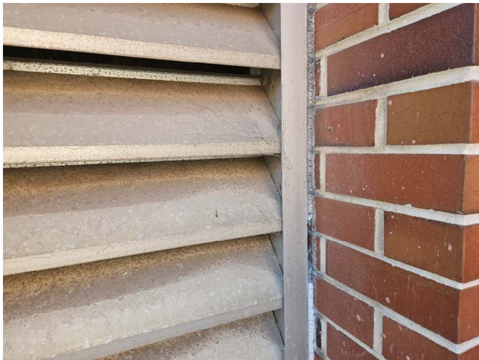
Example of exterior vent with PCB's
