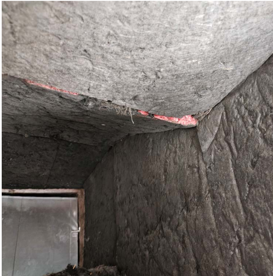
Example of internally lined duct with PCB's <50 PPM
