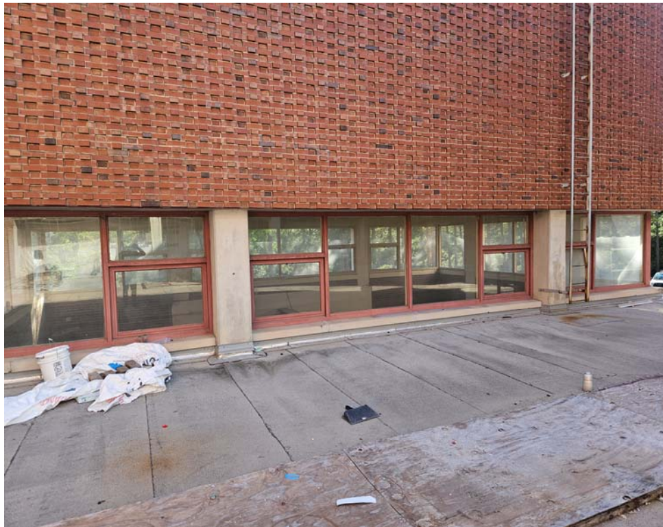
Example of window frames with PCB's and asbestos-containing glazing
