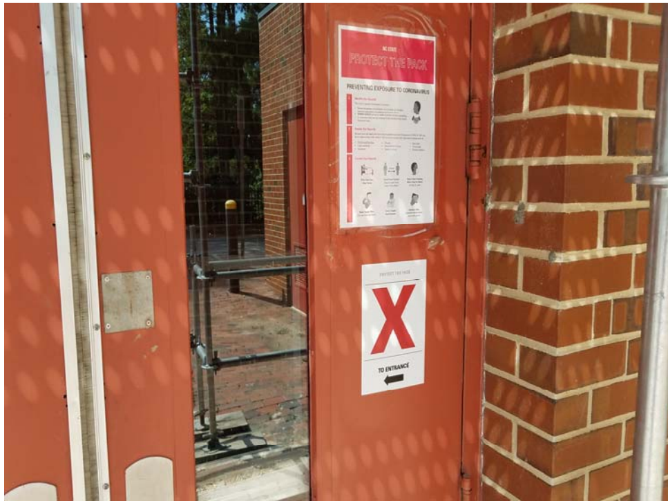
Example of exterior of door with PCB containing caulk
