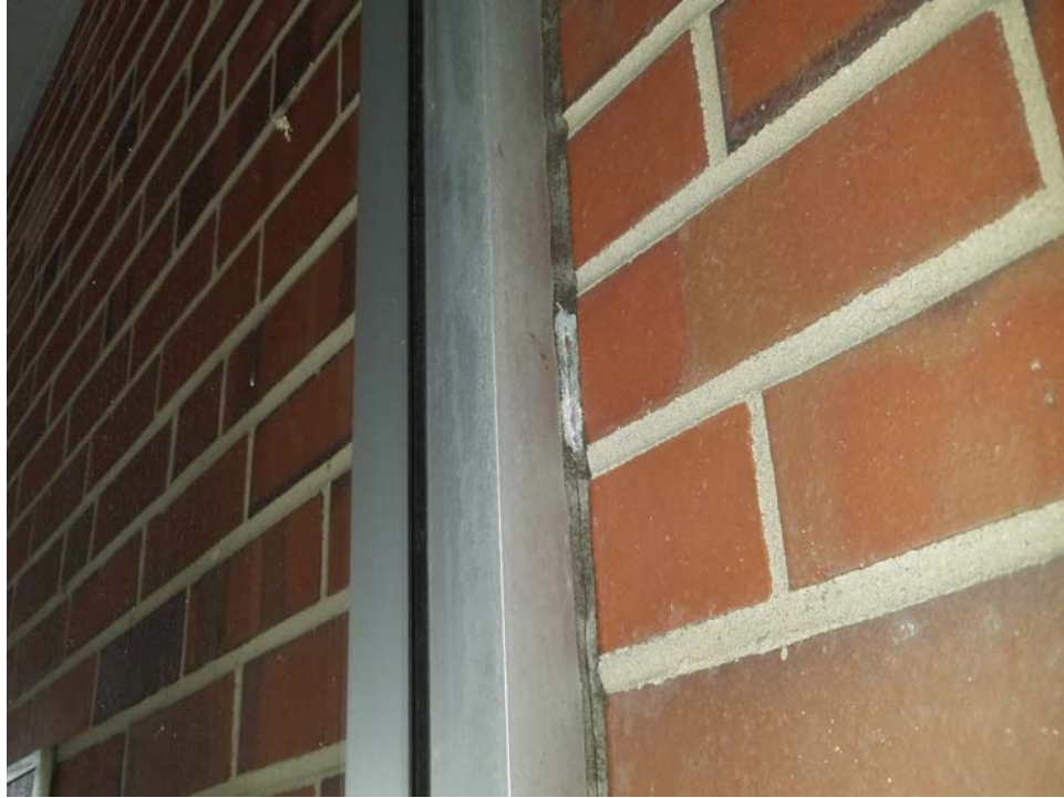
Storefront door complex with asbestos-containing and PCB containing caulk
