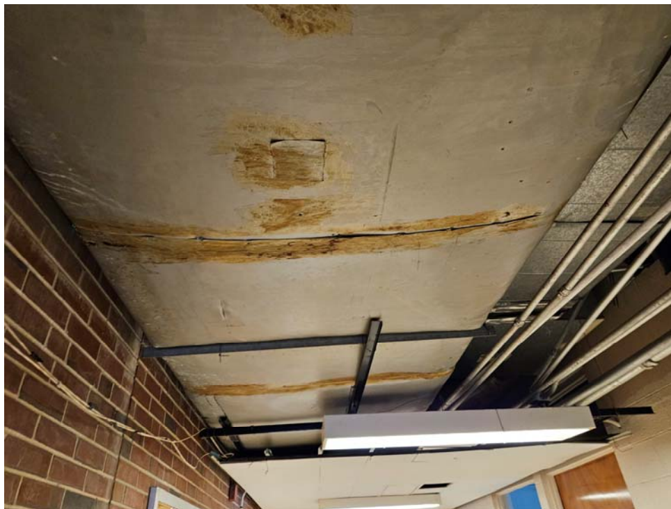
Example of duct with PCB containing mastic/glue
