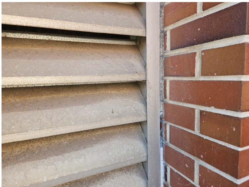
Example of exterior vent with PCB's
